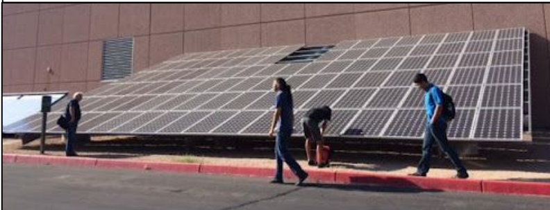
Solar research facility at ASU Research Park used for experiments and data collection.
