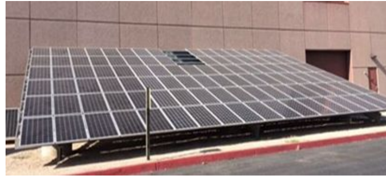
ASU Solar Array with Smart Monitoring Devices
