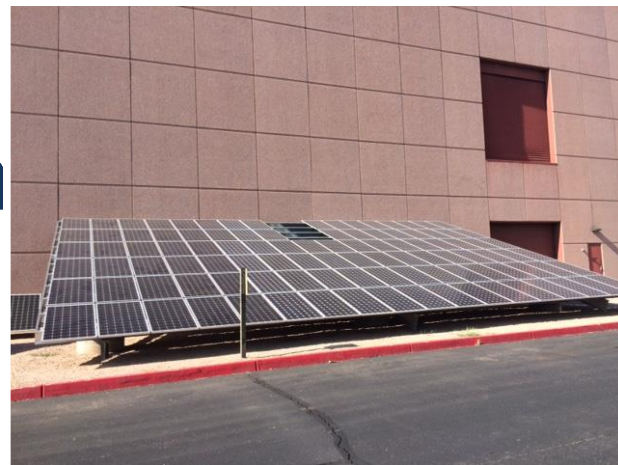
SenSIP -13x8 Solar Facility @ ASU Research Park.
