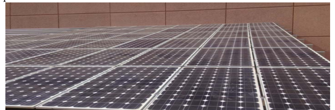
Figure 2. The SenSIP PV experimental facility [1] used to validate our CPS algorithms for fault detection.
