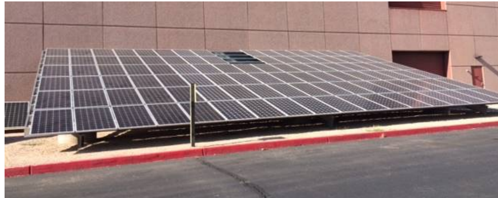
Solar Monitoring Facility at the ASU Research Park.
