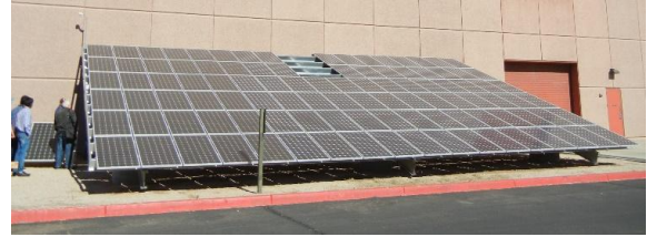
Fig. 3. Utility-scale Solar Array Testing Facility.
