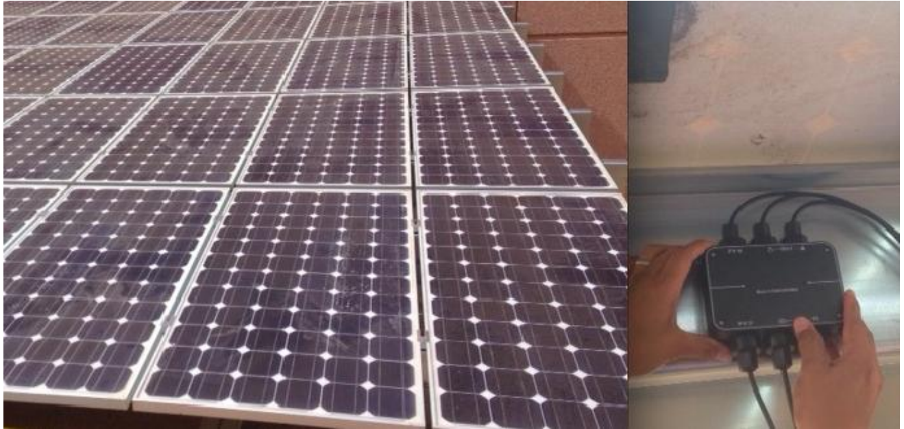
Fig. 2 104 (8x13) Solar Panels installed producing roughly a total of 18kW. Each panel can be monitored individually and all data is transmitted to a server. These panels are already installed in the area of Fig.1 marked with a blue rectangle. The facility will become operational in Oct. 2015 after all communications hardware infrastructure is finalized.
